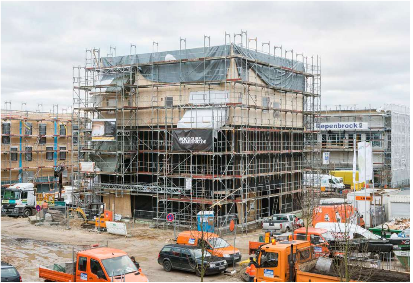
The Woodcube was built using prefabricated wall and floor/ceiling panels. During construction and until the roof was in place, the assemblies were kept dry using tarps and scaffolding.
