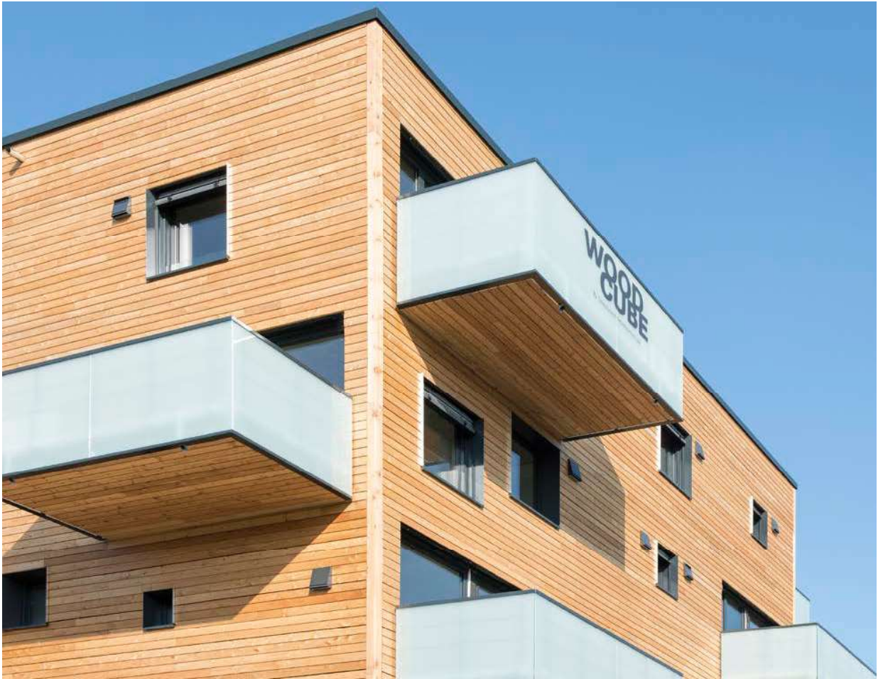
The CLT panels extend the full length of the balconies to provide structural support.
