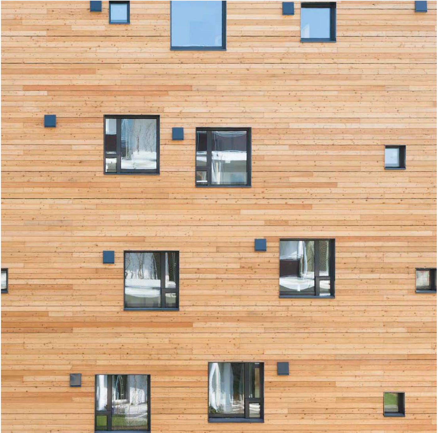
The exterior is clad in unfinished, horizontal larch siding; note the exhaust vents and metal lines indicating the fire compartments.
