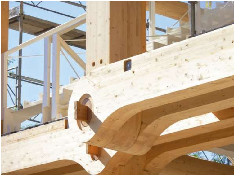
The structural timber frames were assembled on site. Once the frames were lifted into place, installation of floors and walls could begin.
